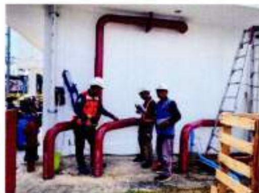
Pipa Hidrant Area Pompa
